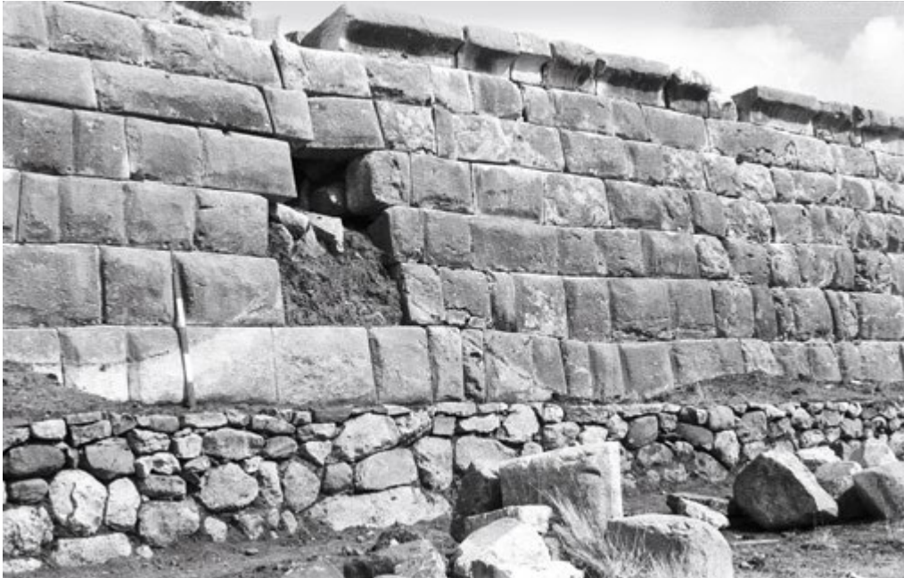
◀ Figure 5 Hole in the masonry of the east wall of the ushnu platform of Huánuco Pampa as it appeared in August 1965 before being repaired by John Murra's team. Rollo 16, foto 7(A), John Victor Murra Archive, Junius Bird Laboratory of South American Archaeology, Division of Anthropology, American Museum of Natural History.
